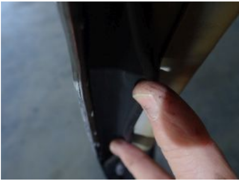
One of the door seals was installed with wrong edge glued down.
