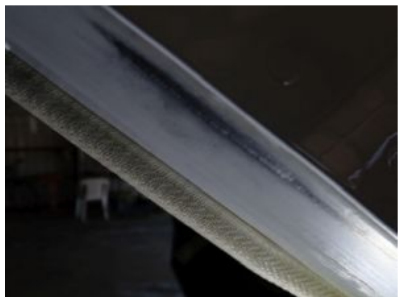
Wear on door frame, adjust the door flange so this no longer wears to avoid future problems.
