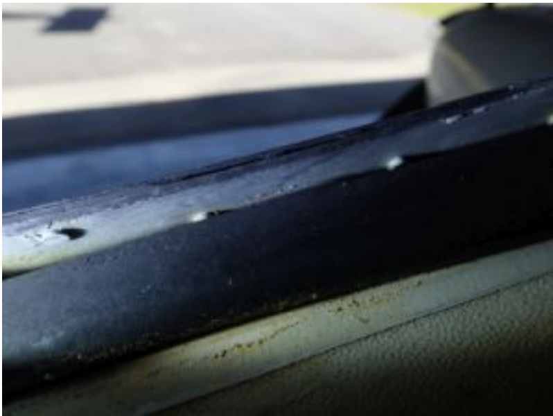
This is the part of the door which needs to be shortened to stop the wear on the frame.
