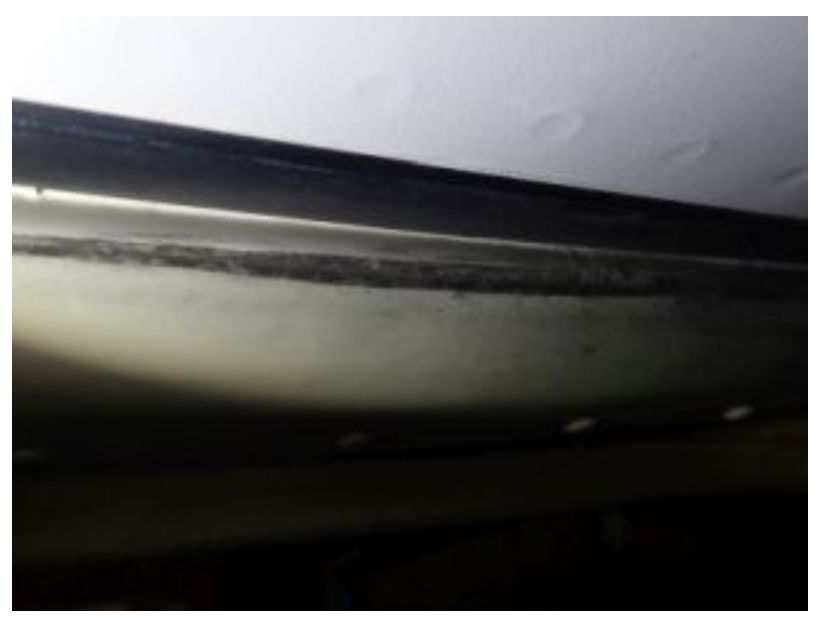
Another wear point on the door frame.
