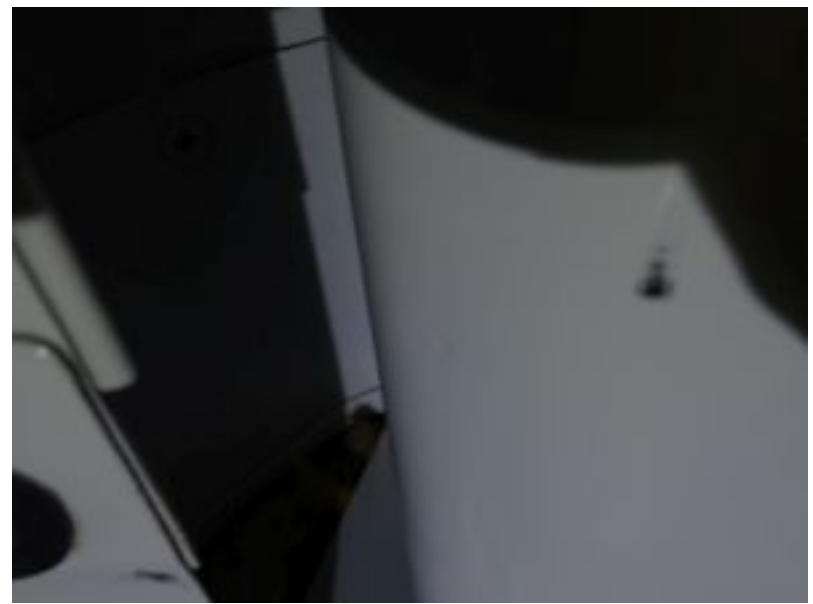
Poor picture of this... long screws in the under-wing gap seal are making dents on the flaps.
