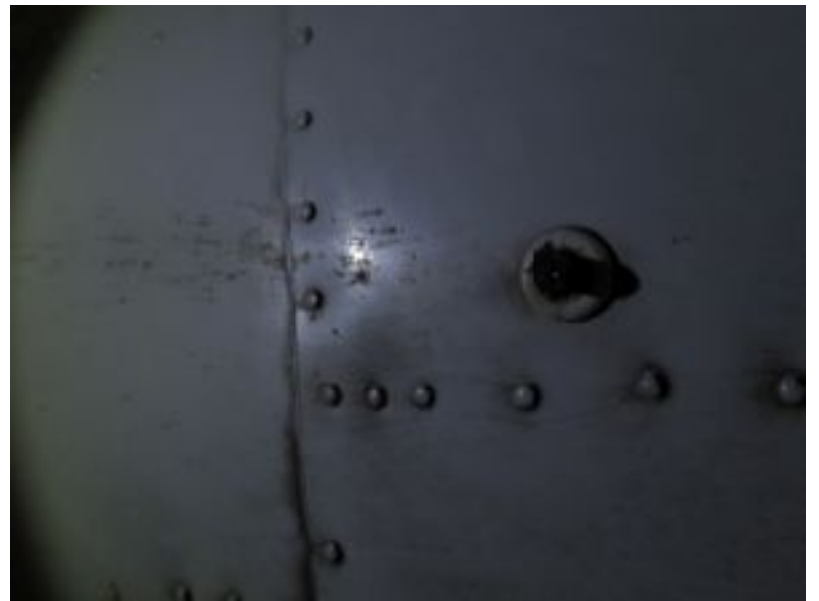
Battery acid is eating the paint behind the battery drain, best to clean it up and protect it.
