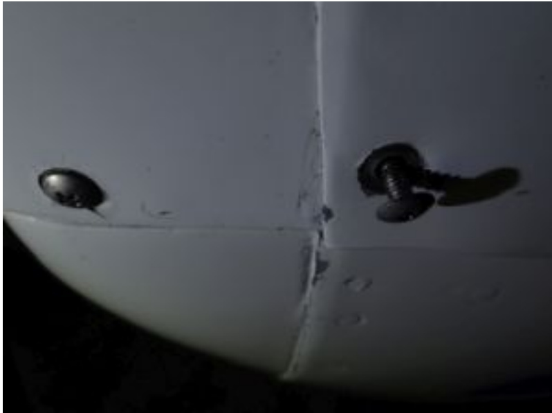
Machine screw where most have a sheet metal screw, but the proper receiver was installed so it is OK.
