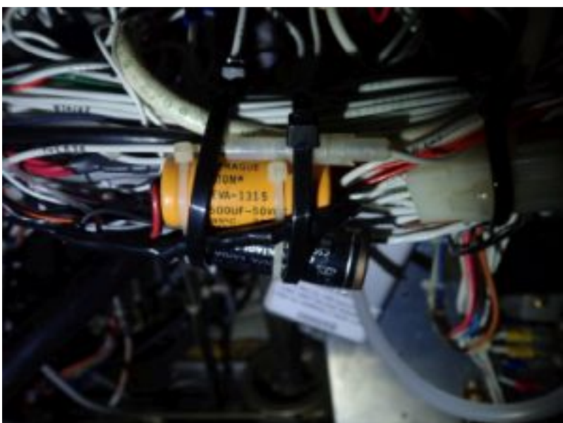
Over Voltage switch is installed, could cause trouble later. Just remember it is there so you'll know where to look when trouble comes.
