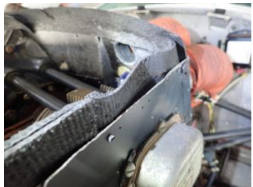
Engine baffle seals are wearing into the cowl, should be protected with aluminum duct tape or epoxy paint.
